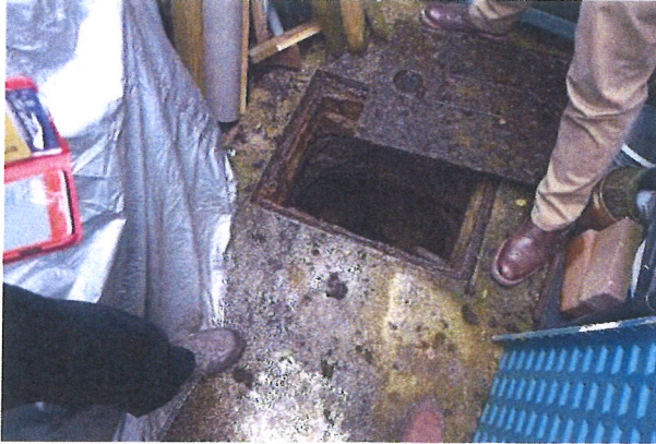
D-23 Dug-well at Riverdale: well-head
